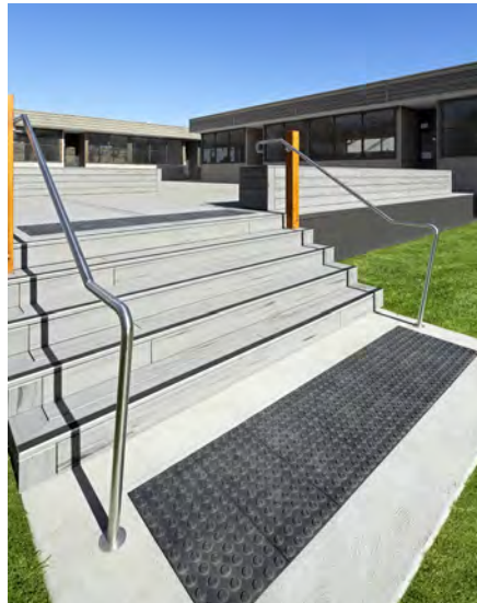
DTAC Ultimat ® Tactiles and Urban Stair Nosing installed at stairs to demountable area
