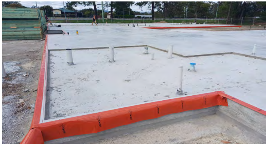
Perimeter installation prior to the standing of the frames. The Kordon termite system has been installed for light weight cladding on the right and a cavity brick installation on the left. This illustrates Kordon's flexibility and adaptability
