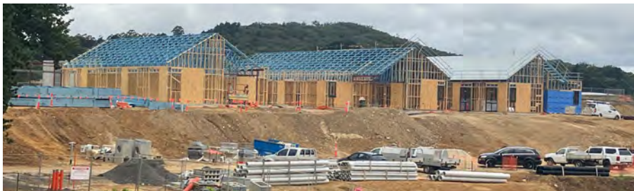
Prefabricated roof trusses assembled offsite at Stratco X1 for precise and efficient installation
