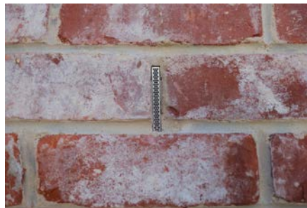
Stainless Steel Weepa in brick wall
