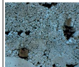
Poor quality concrete – Honeycombing and timber.
